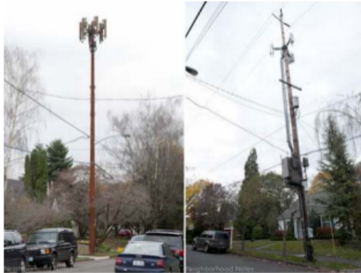
Cell towers can be varied in their height and appearance.
